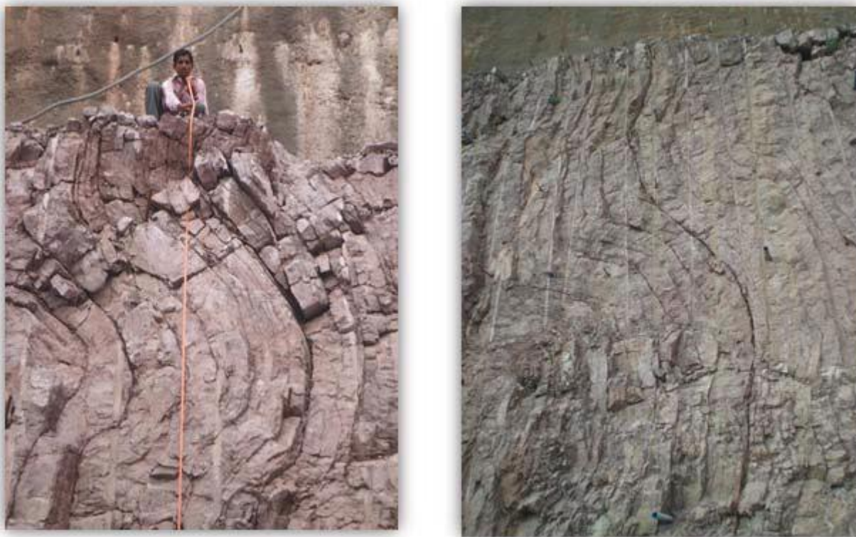
Figure 10 - Photographs showing joints and folding in the rock mass at Approach Channel Area
