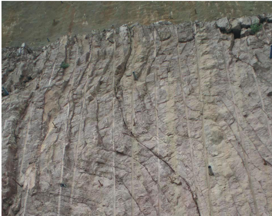
Figure 14 - Photograph showing improvement in pre-split blast results at crest portion of bench
