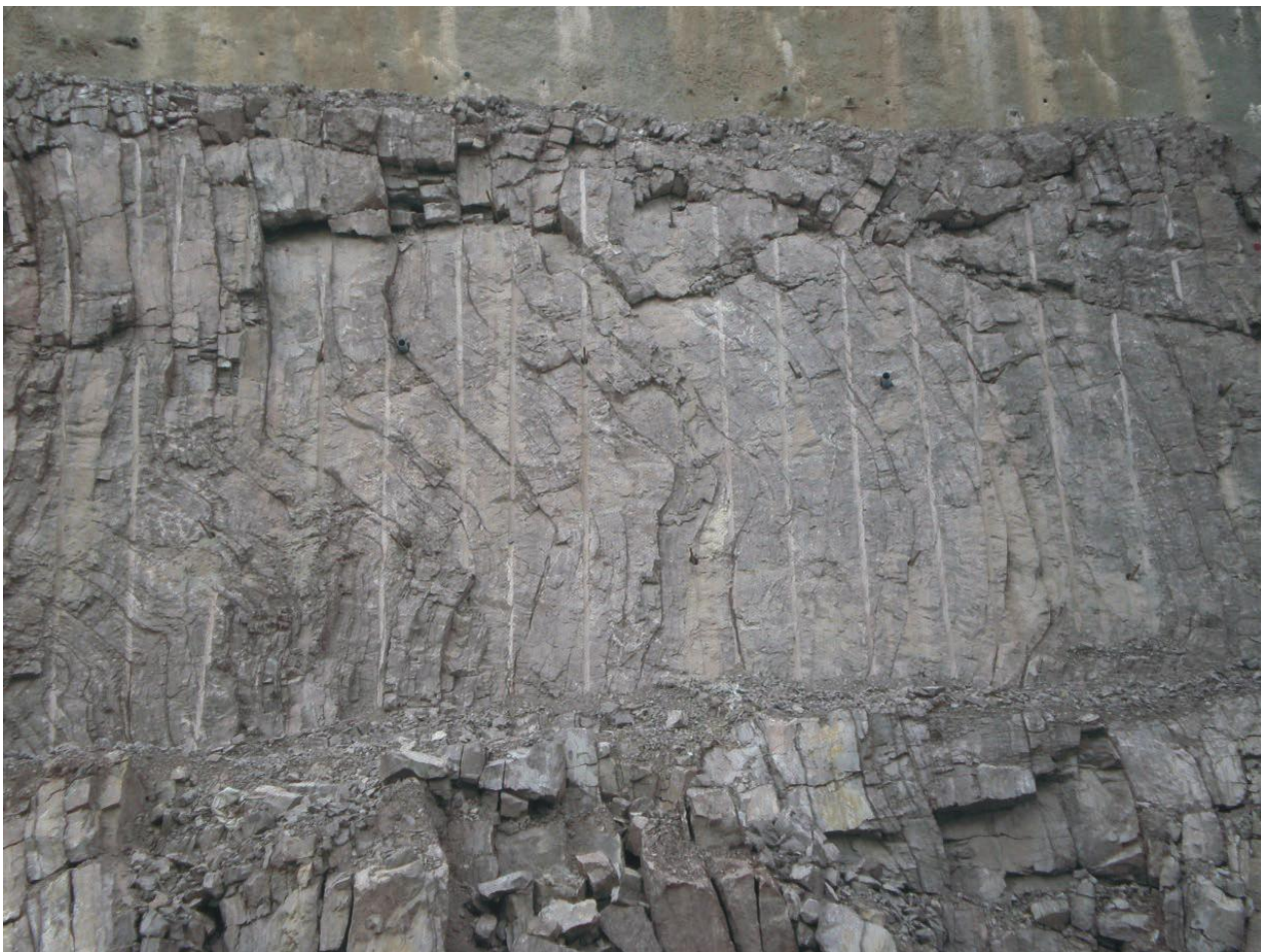
Figure 12 - Damage in the crest portion of the rock mass due to sub-grade drilling
